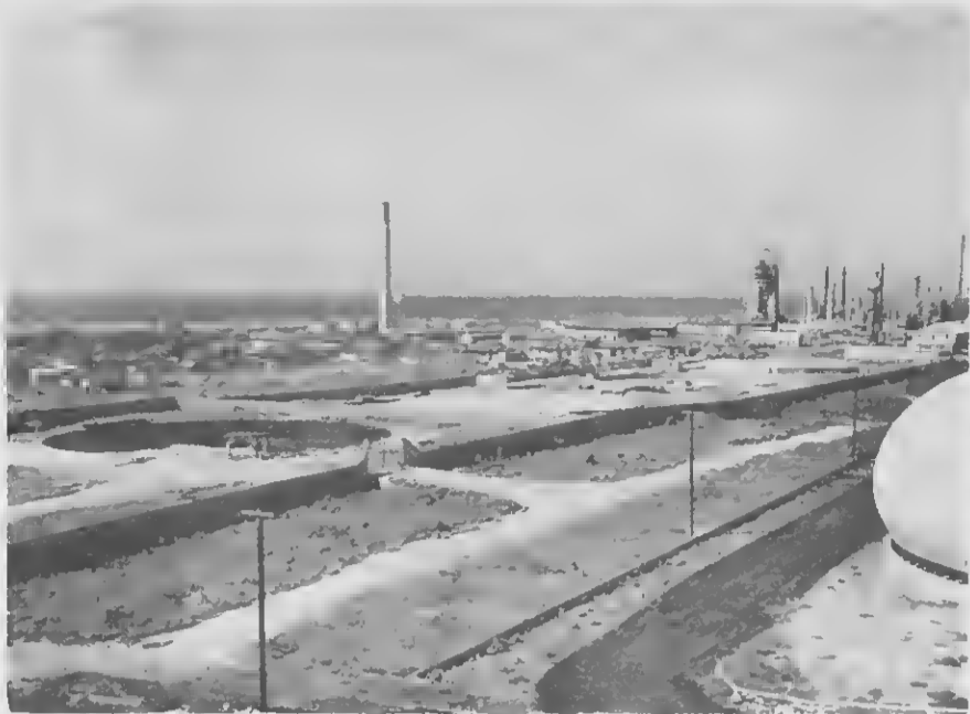
THE GROUND is cleared and bottoms are ready for the erection work to begin. This sequence of photographs shows construction progress on a E SUELO ta worde limpiá y prepará pa e trabao di ereccion cumianza. E secuencia di retrato aki ta muntra progreso di construccion ariha hen-
